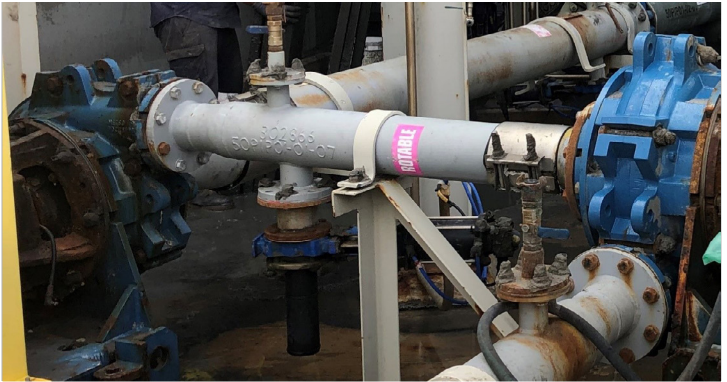
Tails line with two heavy duty HR pumps at Mungari - changeouts now saving 120 hours' manpower per annum
