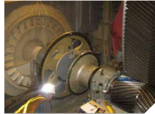
Field personnel align the synchronous motor to the pinion
